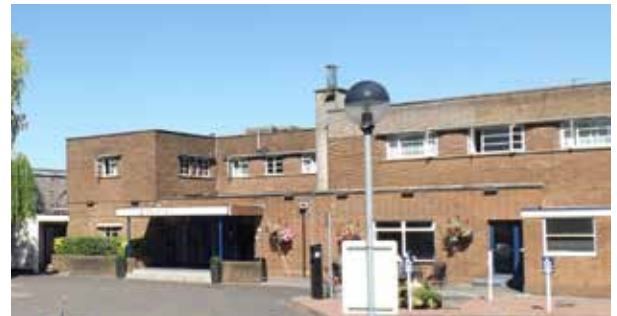
Unsympathetic extensions and additions have been added over time including a small extension to the side of the main bar, and the infilling of the rear courtyard and creation of the reception area.
