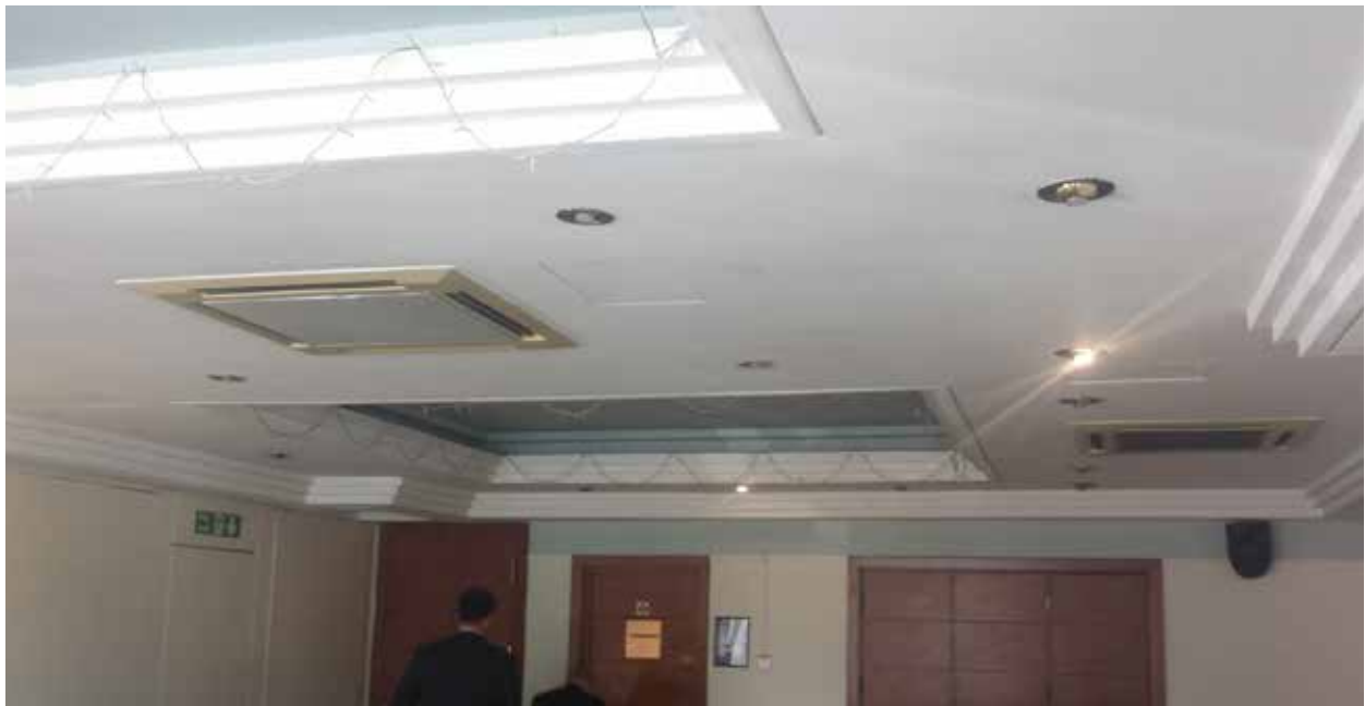
Example of lowered ceiling, installed during a previous refit (prior to listing). Above the suspended ceiling, all trace of former finishes has been removed.
