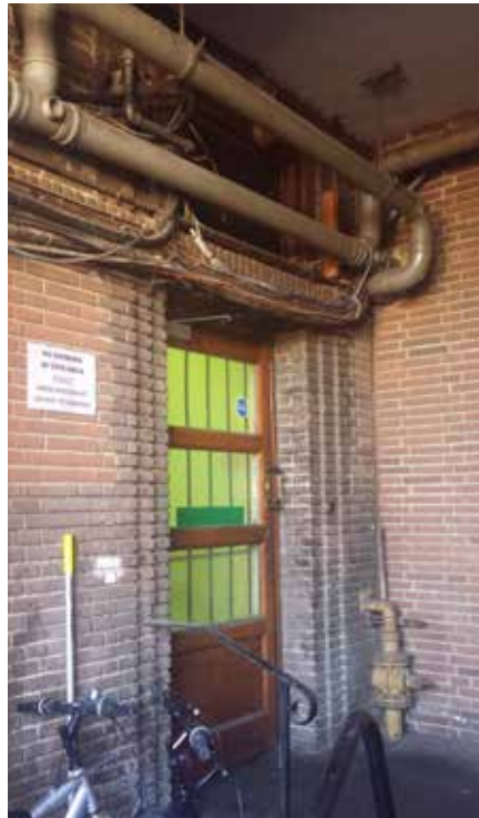
Original entrance from rear yard to building still in situ although a number of services encroach upon detail.
