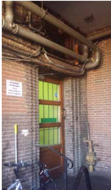
Original entrance from rear yard to building still in situ although a number of services encroach upon detail.
