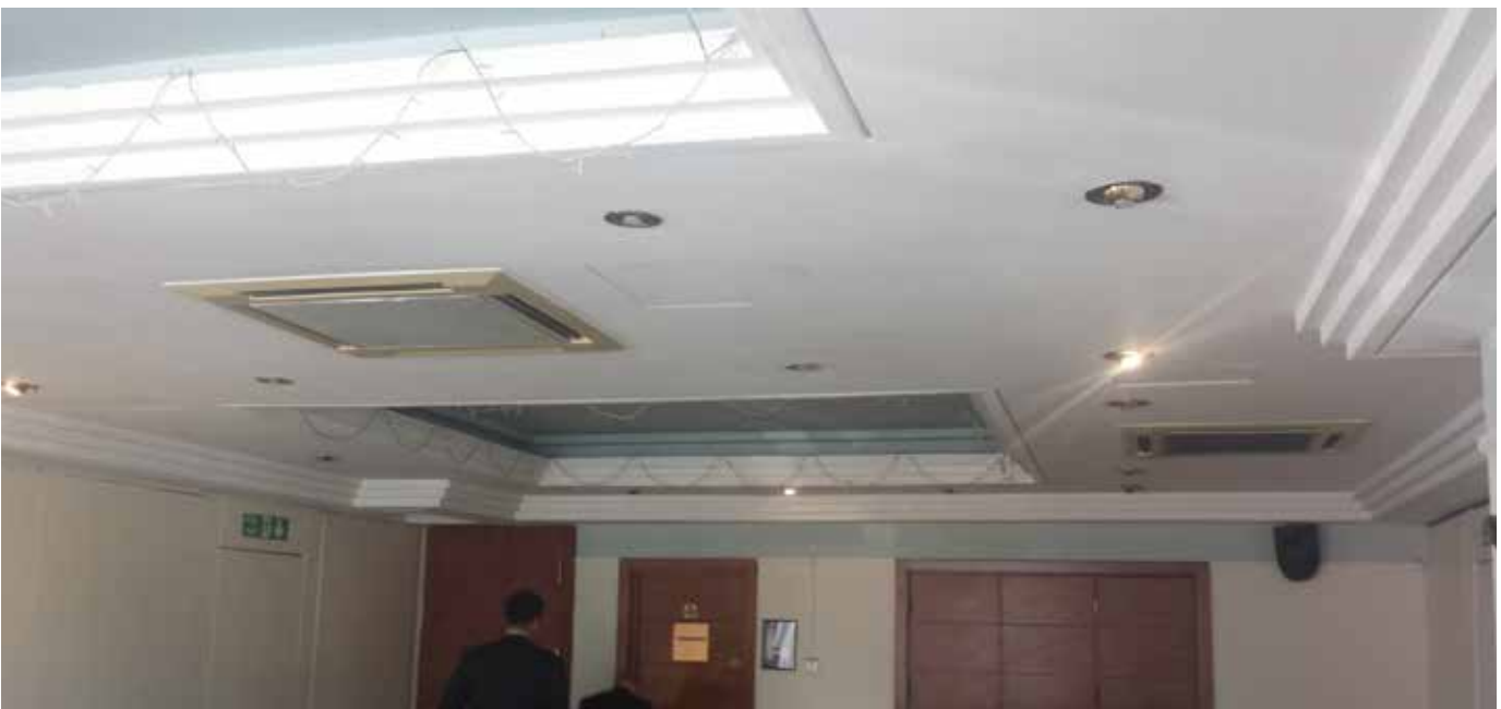
Example of lowered ceiling, installed during a previous refit (prior to listing). Above the suspended ceiling, all trace of former finishes has been removed.
