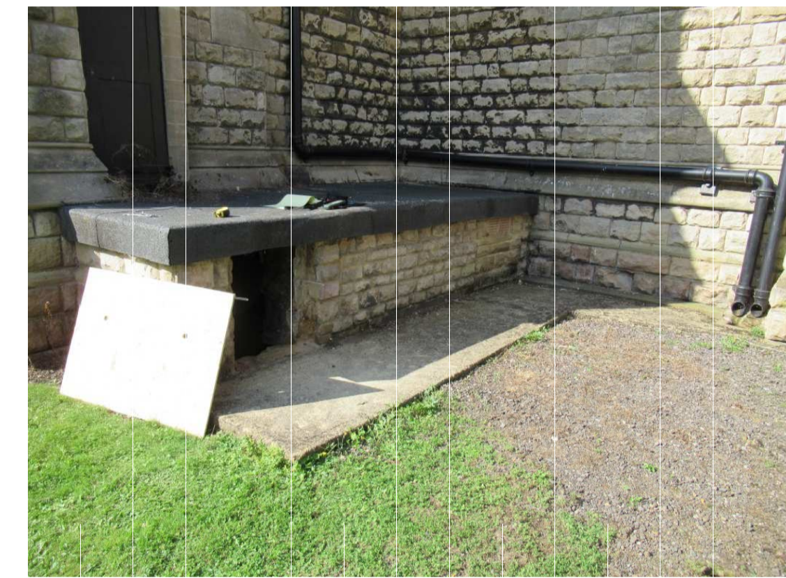
○ IMAGE OF REDUNDANT BOILER ROOM
