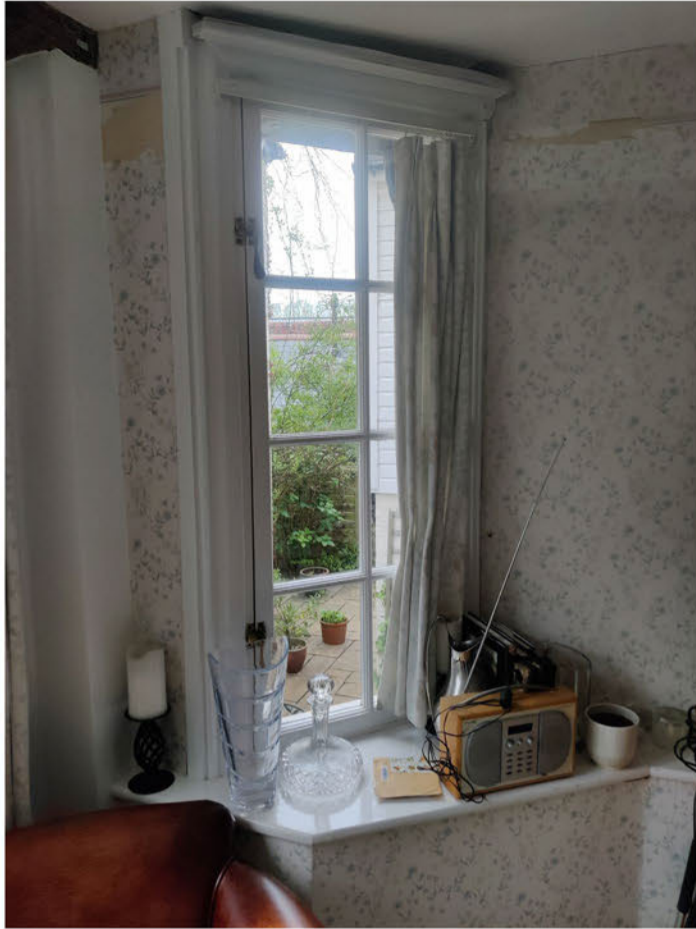
ITEM W16 - CASEMENT WINDOW OPENING IN. THE FRAME IS IN GOOD CONDITION AND CAN REMAIN. NEW CASEMENT LEAF FITTED GLAZING PATTERN TO MATCH EXISTING. CURRENT GLAZING BARS 25mm WIDE, NEW TO BE 24mm WIDE. CURRENT GLAZING IS SINGLE GLAZED, NEW DOUBLE GLAZED WITH A SLIMLINE WHITE SPACER. PAINTED WHITE SASHES AND FRAME EXTERNALLY AS EXISTING.
