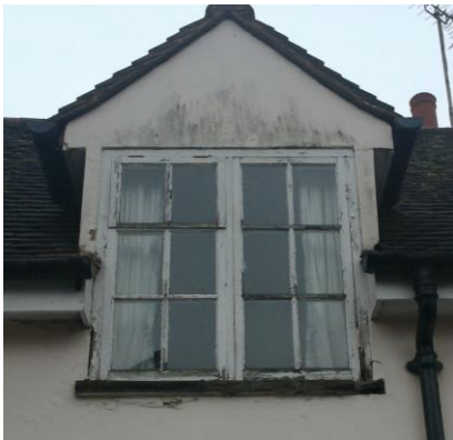
Figure 1 – front upstairs left
