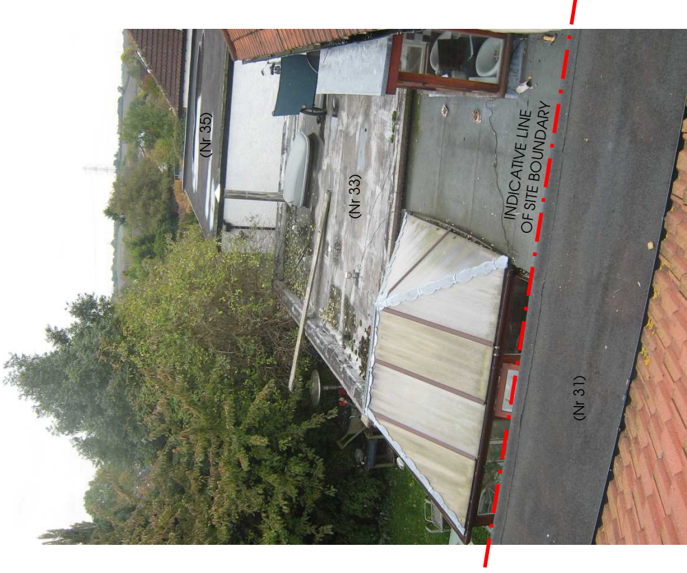
VIEW FROM LOFT ROOM ACROSS ROOF OF EXISTING GARAGE (Rear roofscapes of 33 and 35 Northaw Road East beyond)
