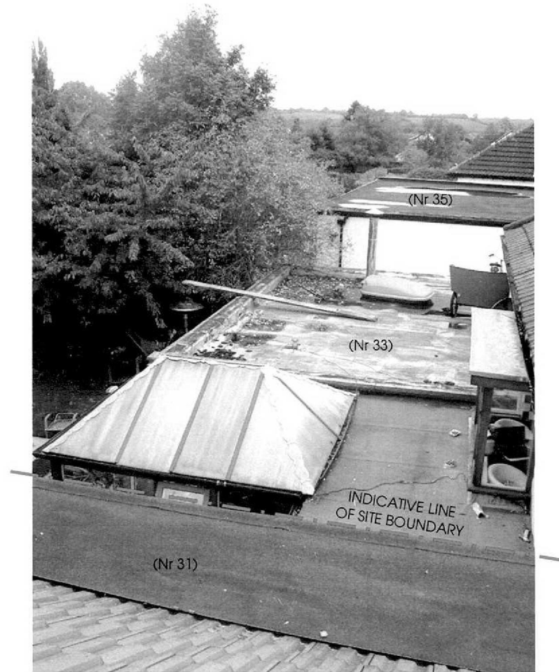
VIEW FROM LOFT ROOM ACROSS ROOF OF EXISTING GARAGE (Rear roofscapes of 33 and 35 Northaw Road East beyond)
