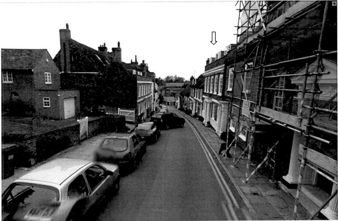
Photo 7: Streetscene view of Fore Street showing site context. No. 16 is on the right hand side of the picture.
